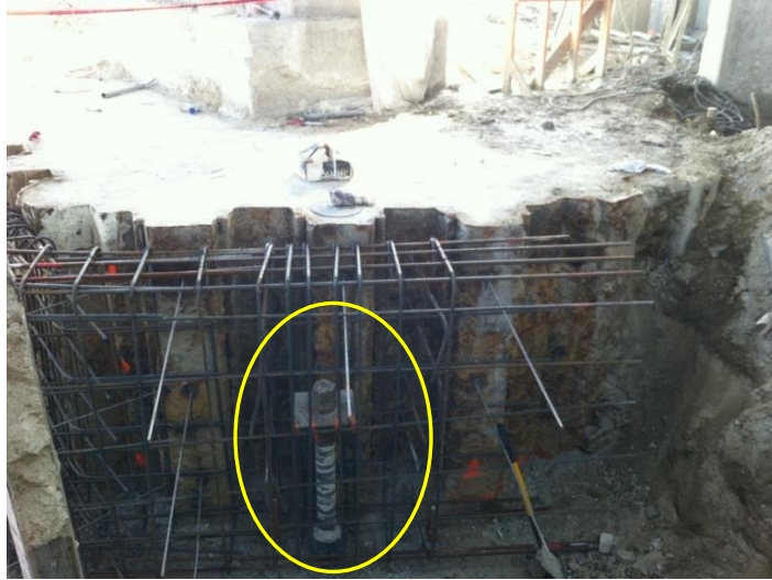
Figure 8. A view of an installed underpinning micropile on the north side of pier G-18 prior to pilecap expansion
